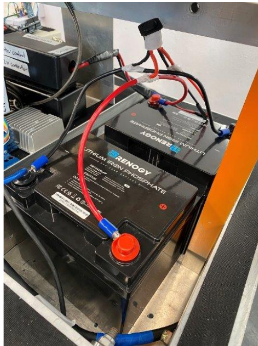
Figure 5: Batteries wired in parallel
