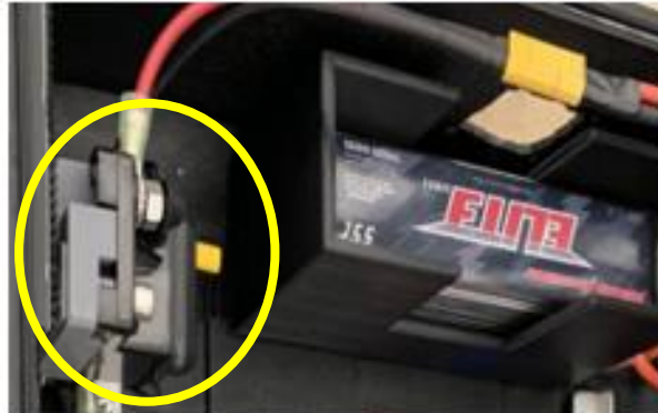
Figure 2: New Circuit Breaker
