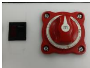
Figure 5. Dual Power Switches.
